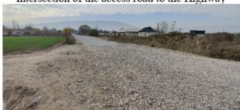
Damaged approach of Bridge-1
