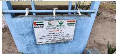
Water Tape at the Medical Centre Compound
