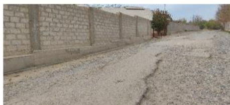
Damaged Paved Road
