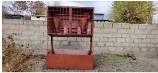
Unused & unlabelled Fire extinguisher at the Medical Centre compound
