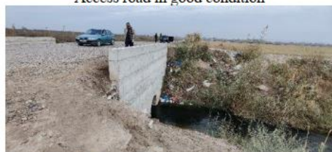
Side view of damaged bridge-1
