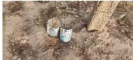
Hazardous empty paint containers are in the Project site
