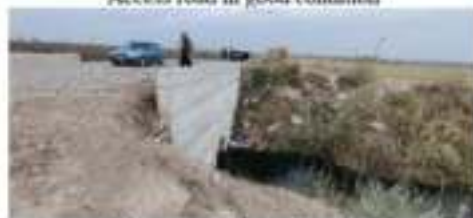
Side view of damaged bridge-1
