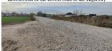
Damaged approach of Bridge-1
