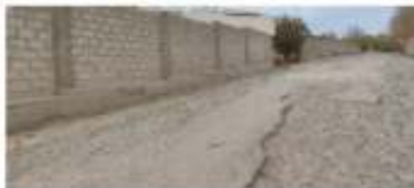
Damaged Paved Road
